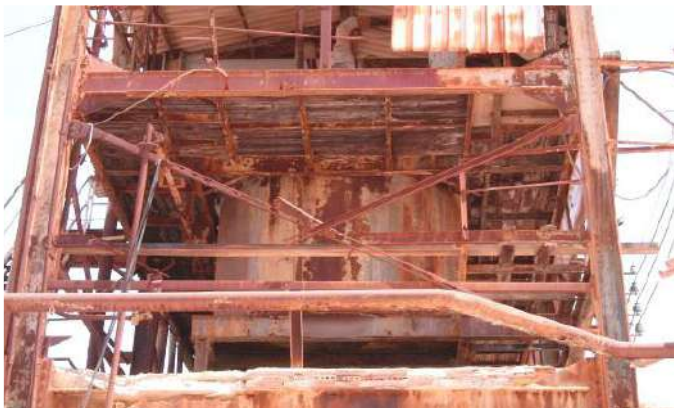
Figure 2 Damage in the bracing system.
