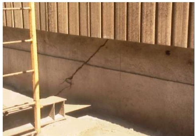
Figure 9 Cracking 45 degrees to both directions and both side of joint.
