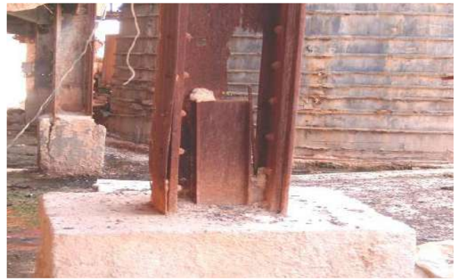
Figure 3 Corrosion of columns.
