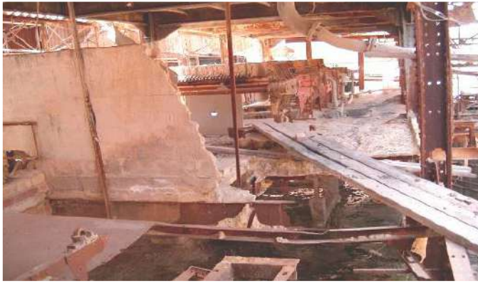
Figure 6 Collapse of a floor.
